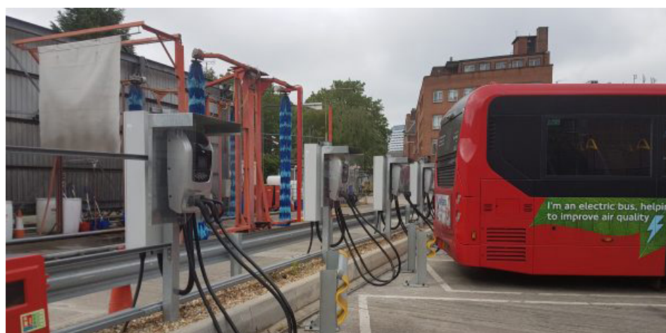
FIGURE 4: AC III E-BUS CHARGERS IN THE UK [SOURCE: (IAN, 2018)]
