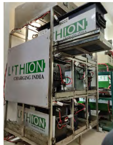
FIGURE 23: LITHION POWER E-3W BATTERY SWAPPING INFRASTRUCTURE
