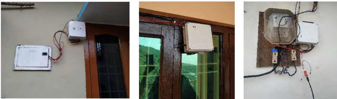
Figure A.1.13. Smart energy loggers installed at site
