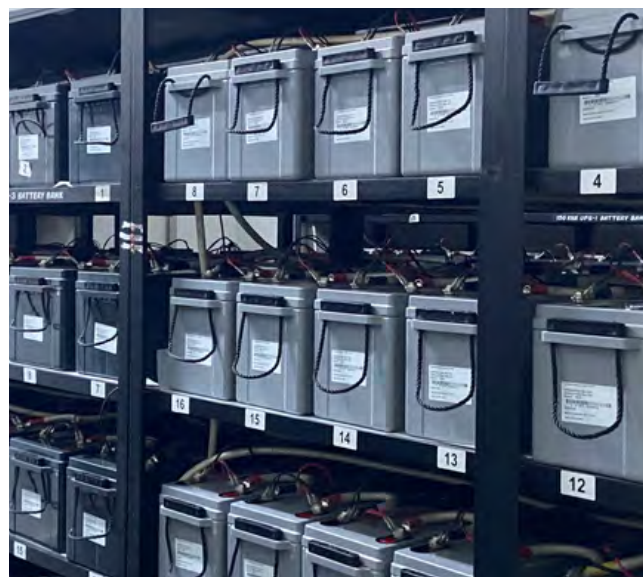
Figure 5.5: Modular UPS battery bank
