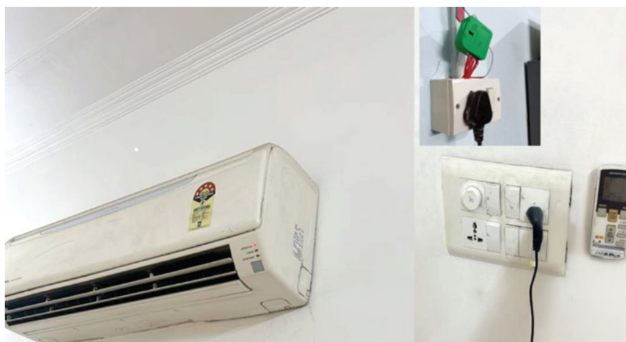
Figure 4: LoRa system installed on the customer's air conditioning unit
