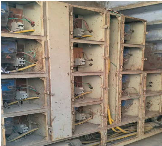
Figure 15: Electric meter boxes exposed because covers stolen
