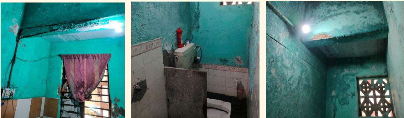
Figure 7: Seepage and moisture on interior walls, ceiling, toilet in a home
