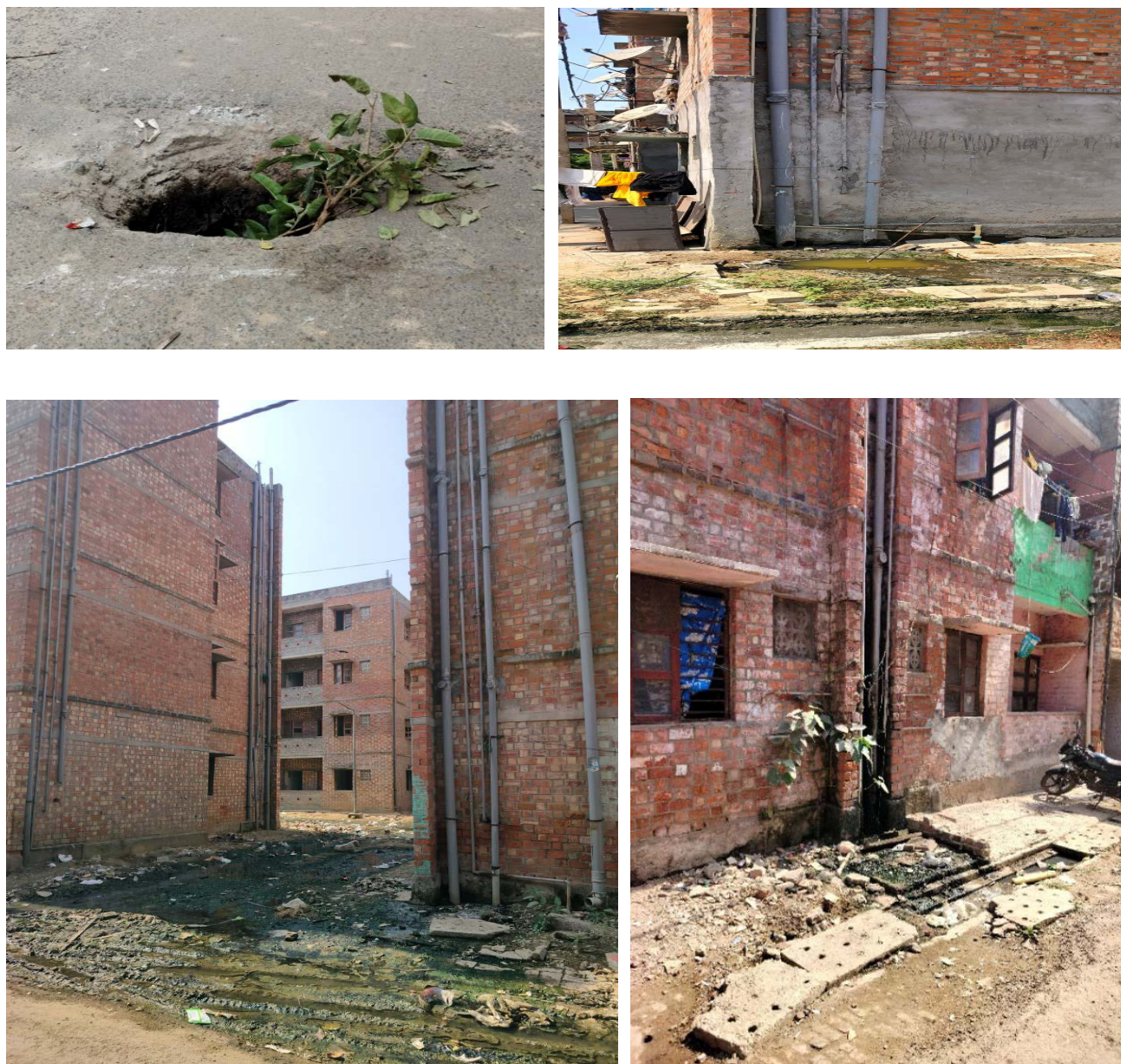
Figure 12: Overflowing sewage and storm water drains, missing/broken drain covers
