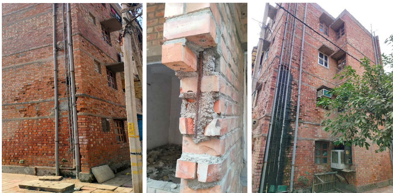
Figure 9: Seepage on external walls, deterioration of bricks
