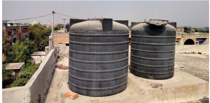
Figure 14: Water tanks unused on terrace
