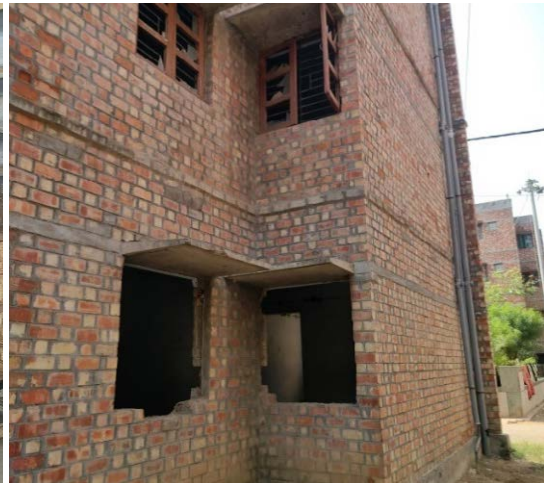
Figure 16: Windows & grills stolen from unoccupied flats
