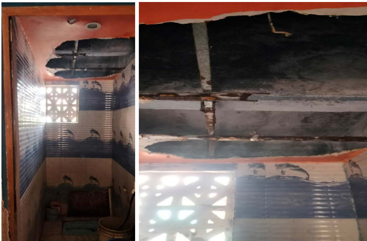
Figure 8: Deterioration of ceiling due to seepage
