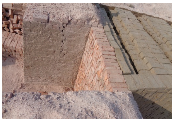
Figure 16: Wicket gate closing with single brick thick wall result in air leakages from gaps between the bricks
