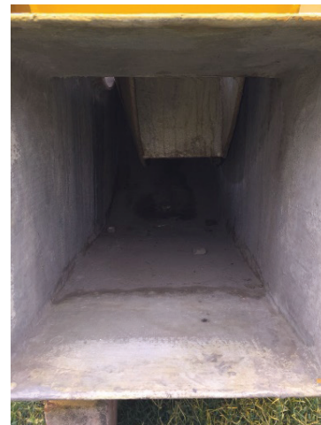
Figure 40: Polymer coating on inner side of fan duct
