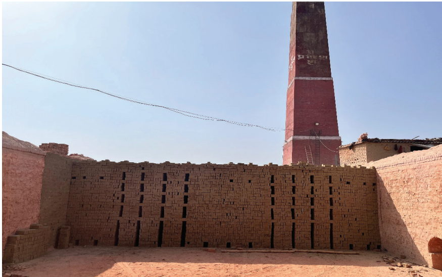
Figure: Double Zig Zag brick setting: Openings for air flow located on the side of the chamber
